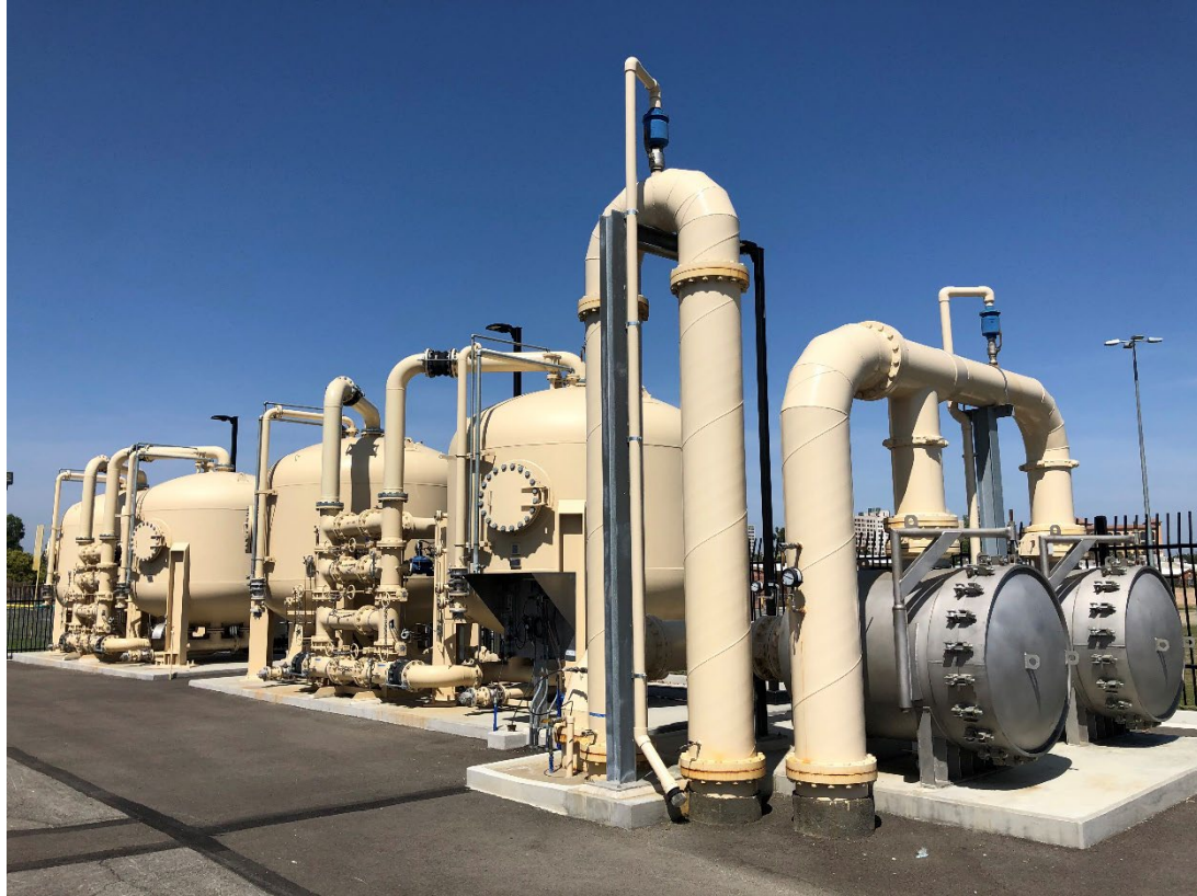
PFAS Equipment at the Westhaven Reservoir
