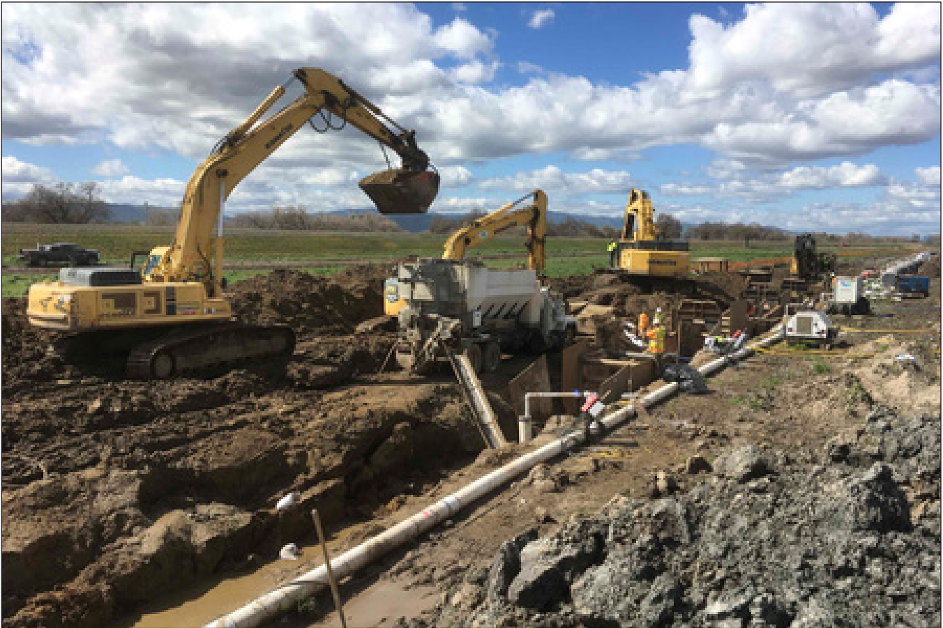
This $28 million recycled water pipeline project was constructed to convey Title 22 recycled wastewater from the City of Turlock's outfall location at the San Joaquin River to the City of Modesto's effluent pump station location about 7 miles away.
