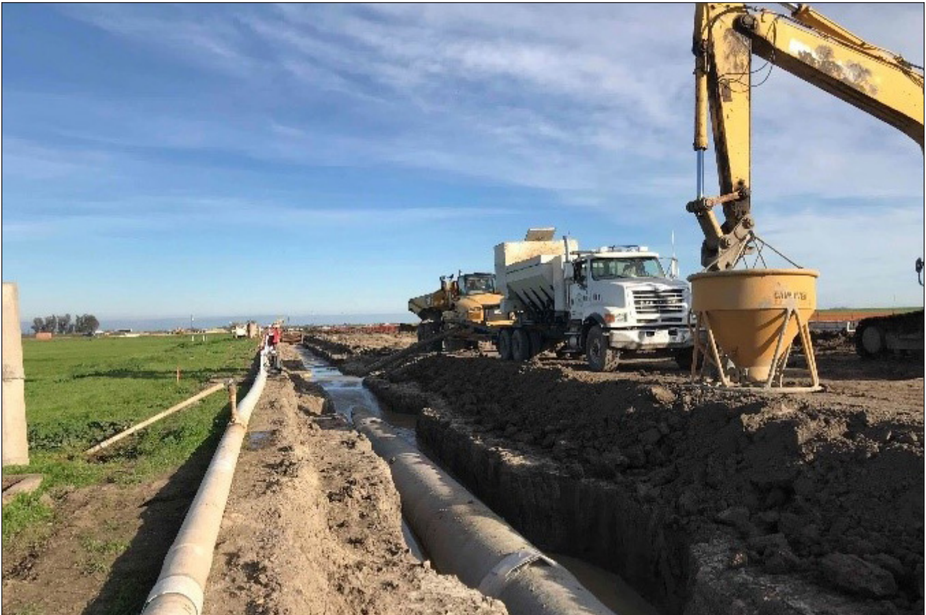
Once completed, Turlock’s recycled water will be pumped from an existing pump station at the City of Modesto’s wastewater plant to the Delta Mendota Canal, where the Del Puerto Water District will extract the water to use for their agricultural needs.
