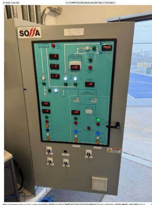
Well 27 PLC Panel
