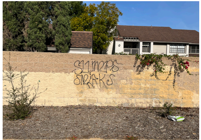
Graffiti on another section of the wall
