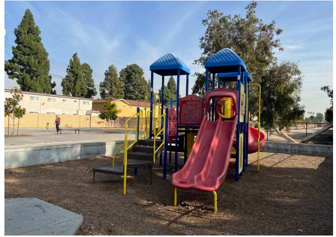
Worn-out playground equipment at the Shelley Kensington Park that is almost two decades old
