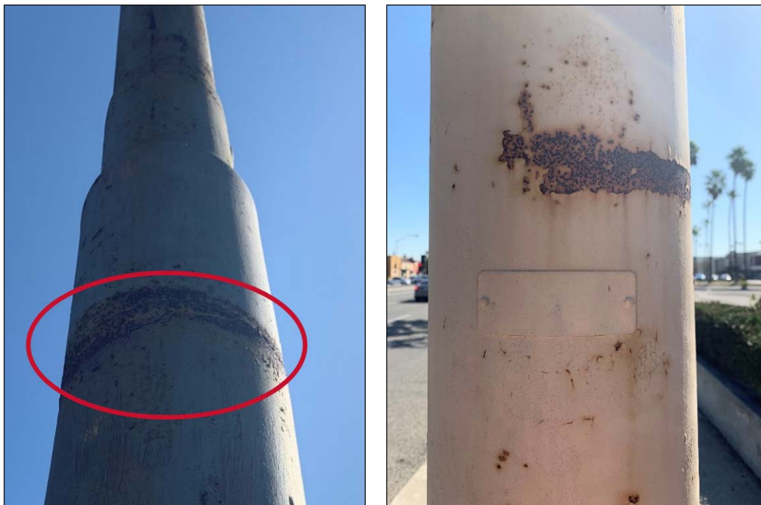
Figure 9 – Corrosion at Weld (Left) and Above Manufacturer's Label (Right), South Banner Pole, Site #4
