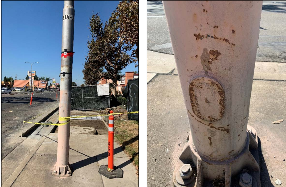
Figure 8 – Corrosion Damage on North Banner Pole, Site #4
