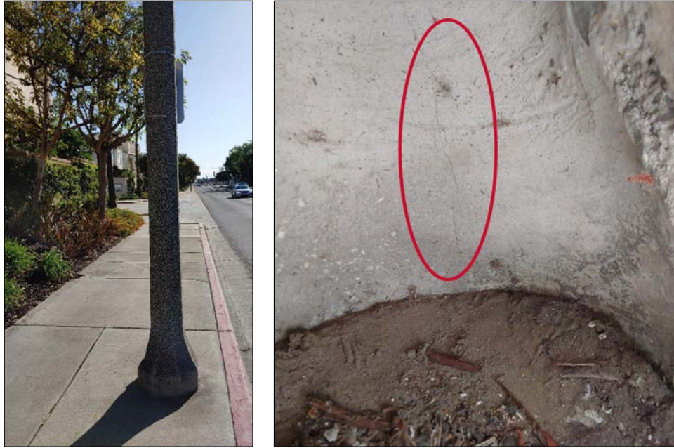
Figure 16 – Interior Crack in North Banner Pole, Site #8
