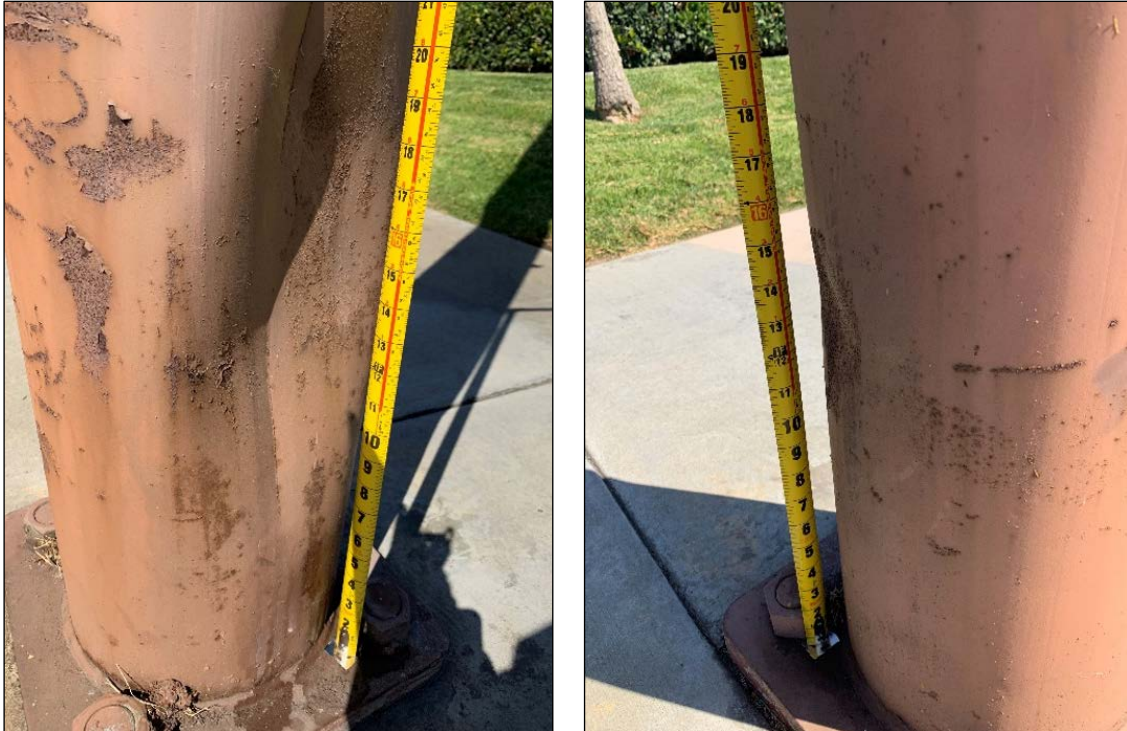
Figure 11 – Dent and Corrosion Damage on North Banner Pole, Site #5
