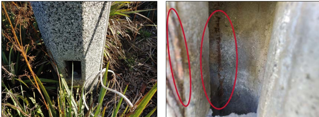
Figure 15 – Corrosion of Reinforcing Steel in Banner Pole in Median, Site #7
