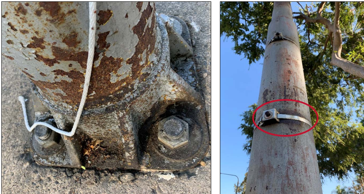
Figure 6 – Corrosion on East Banner Pole, Site #3
