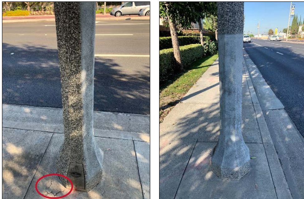
Figure 17 – South Banner Pole, Site #8
