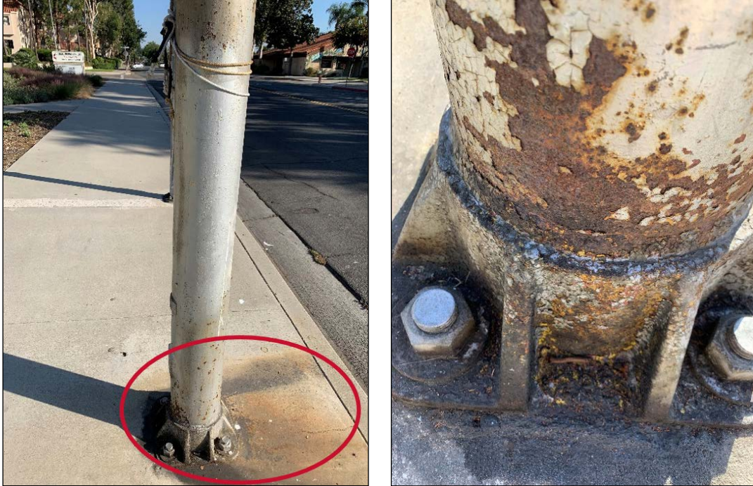
Figure 7 – Rust Stains and Corrosion on West Banner Pole, Site #3
