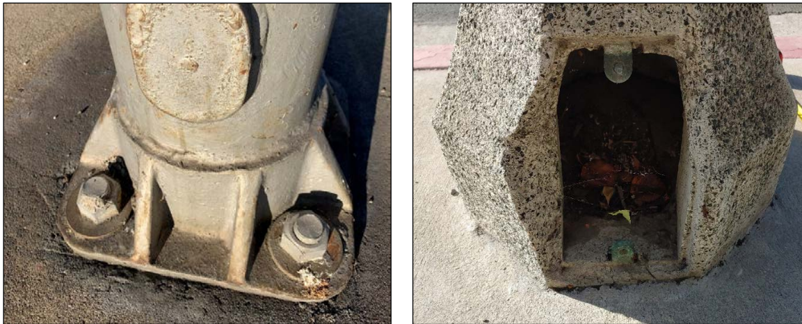
Figure 2 – Flanged Metal Pole with J-bolts (Left), Cast Concrete Pole Embedded in Concrete (Right)
