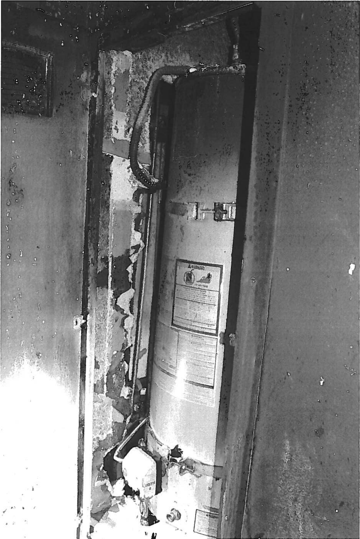
Water Heater 2 nd Floor
