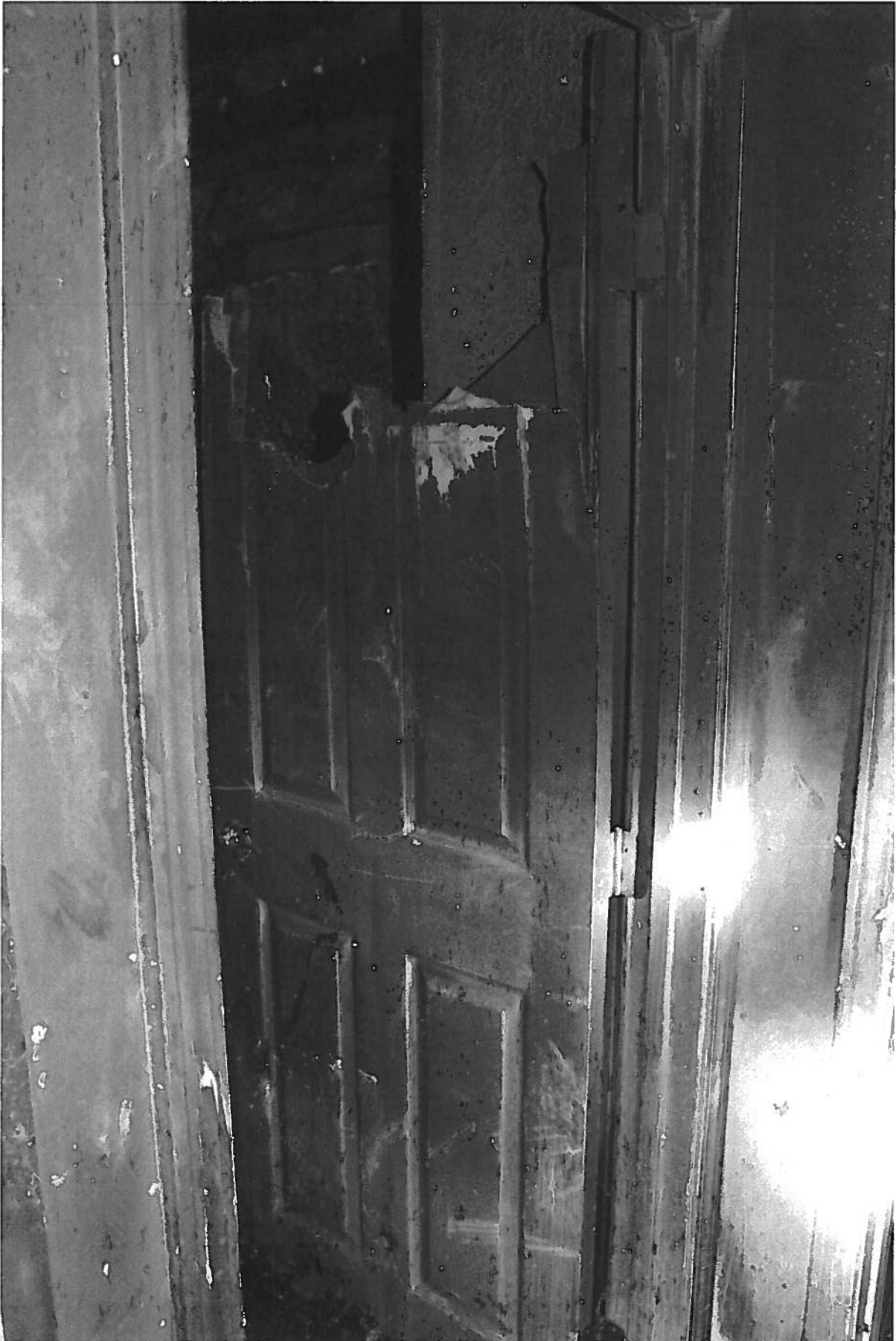
2 nd Floor West Bedroom Door
