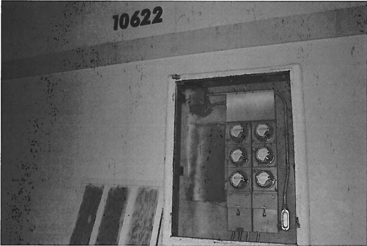
West Wall (Address (numericals only) and West Main Service Panel)
