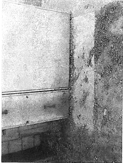
OP06 Close-up view of a utility cabinet.
